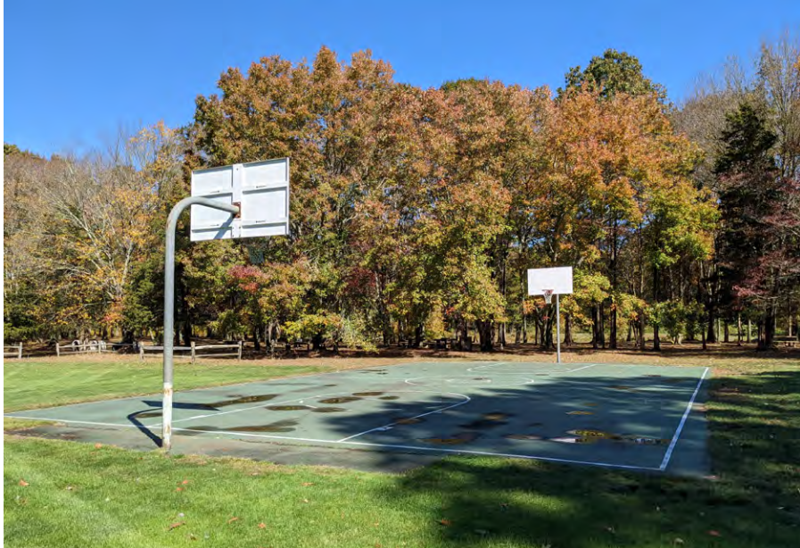
Basketball court: Court is undersized and water puddles on surface.
